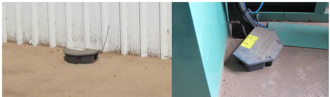
Figure 2: Example of bait stations that are not set properly. Bait stations must be placed against the walls of structures to increase the chance of rats or mice entering and consuming the bait
